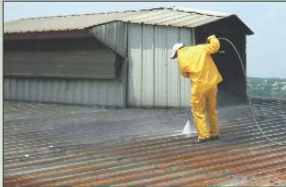
Prepare the roof. Prep and clean the roof, removing dirt and debris.
