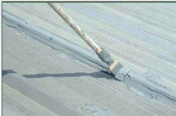
H.E.R. Polyurethane Sealant is applied to the seams, fasteners and penetrations and then smoothed with a brush.
